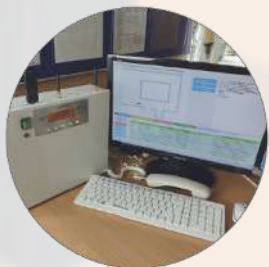
AU TSASPI PPO automatic fire alarm system with phone and monitor display
